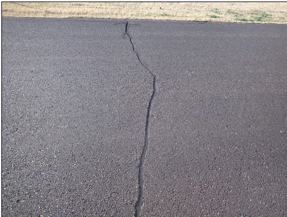
TW-11-01: L&T Cracking
