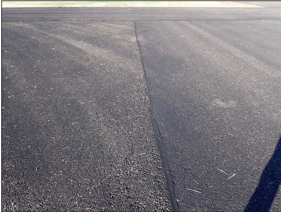
TW-12-03: L&T Cracking
