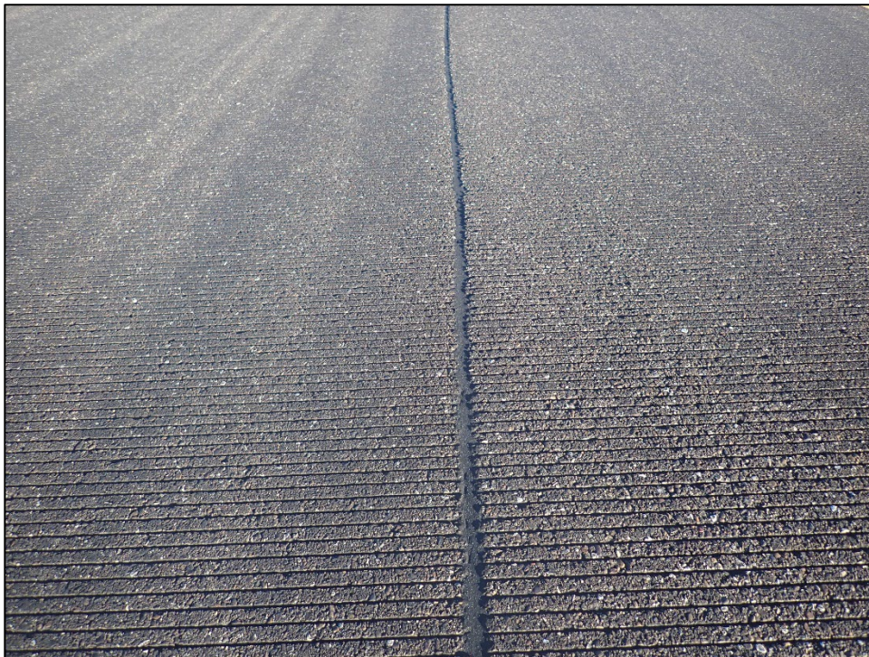
RW11-11-65: L&T Cracking
