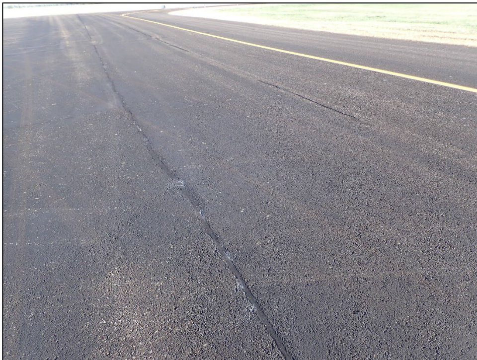
AP-05-06: L&T Cracking
